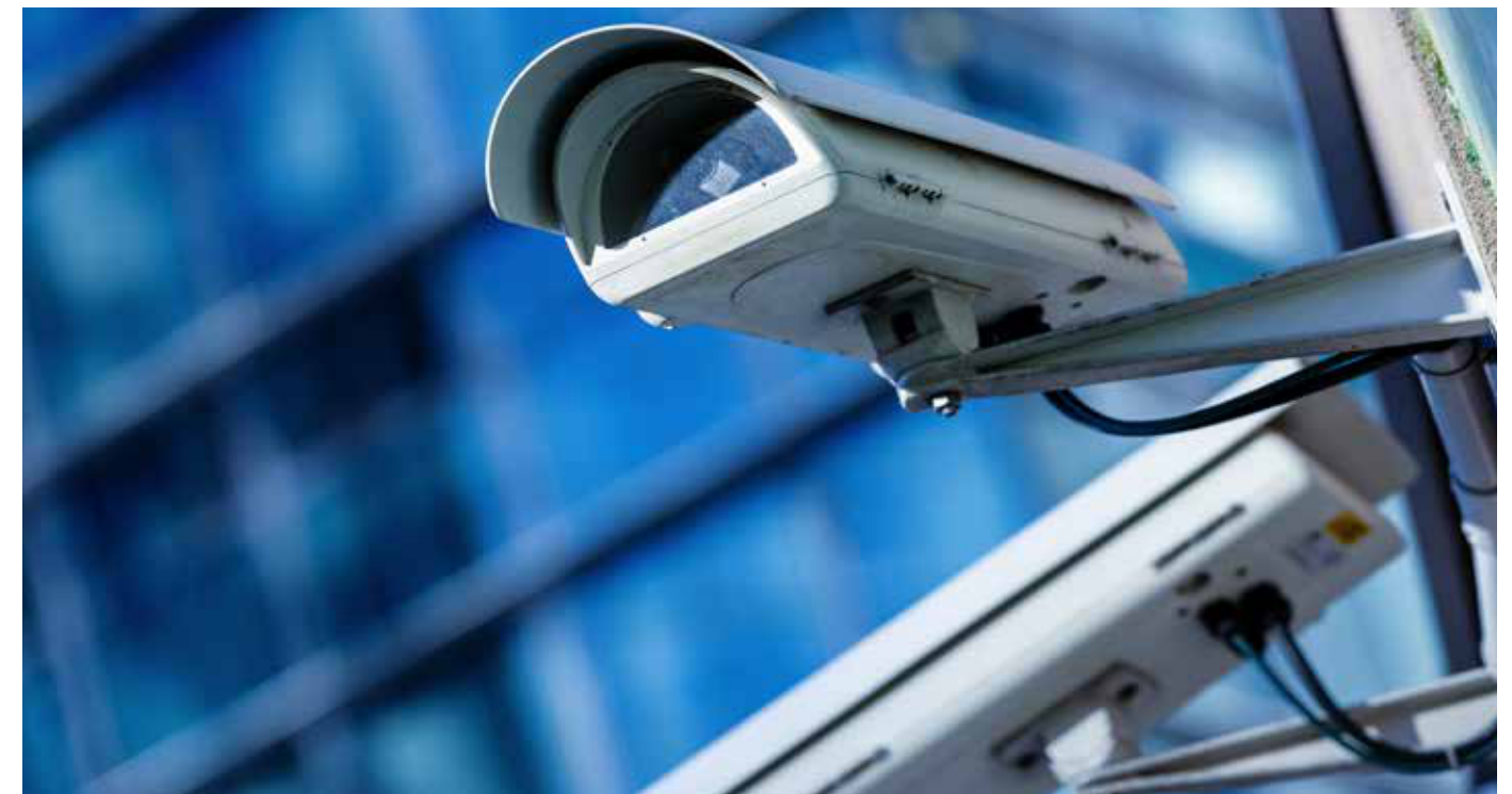
CCTV CAMERA SURVEILLANCE
